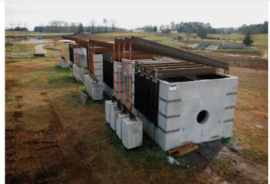
assembled load chambers
